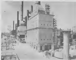
This new furnace for No. 8 Pipestill (in foreground) was placed in service Jan. 24. In background is the furnace of Pipestill No. 7, while the new furnaces for Pipestills Nos. 6 and 5 are scheduled for completion in April.
